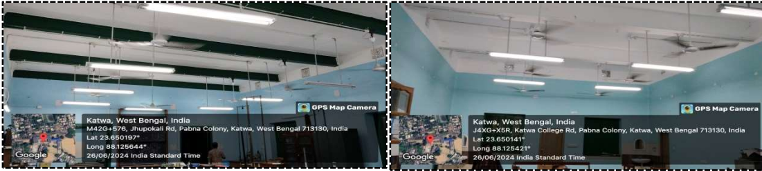
LED facility in the class room
